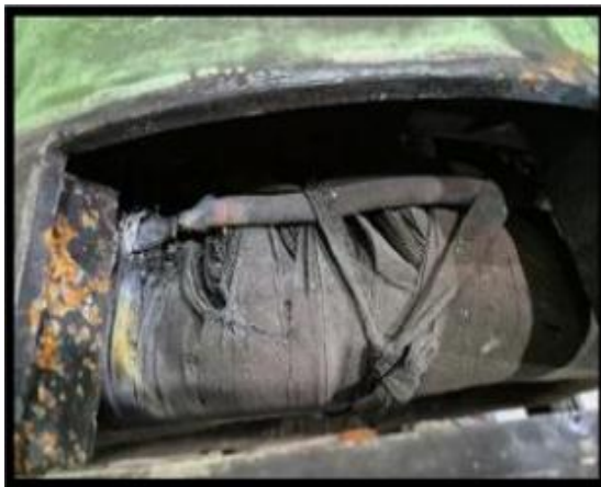
Fig.3 Detail damage stator winding (Burnt winding)
