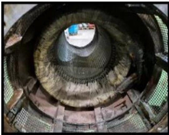
Fig.1 Heavily contaminated stator winding
