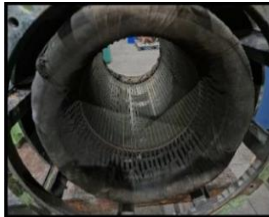
Fig.2 Damaged stator winding (Burnt winding)
